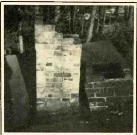
Unit 320 shows us why you should use guy wires on your base station antenna. His antenna, mounted on the chimney, had no guy wires. A wind storm came through town and took down the antenna, along with the chimney. Dean says the impact on the roof sounded like a bomb going off.
